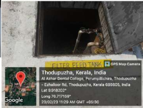
FILTER FEED TANK
