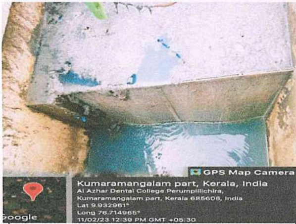
WASTE WATER COLLECTION PIT IN STP
