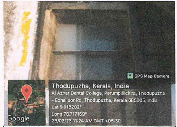
CHAMBER PIT IN STP
