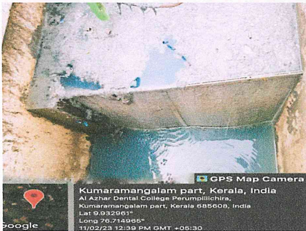
WASTE WATER COLLECTION PIT IN STP
