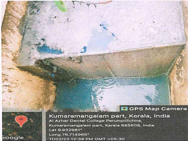
WASTE WATER COLLECTION PIT IN STP
