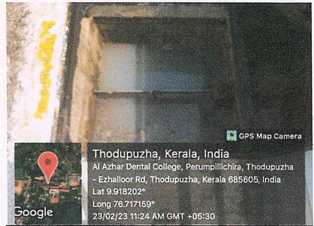
CHAMBER PIT IN STP
