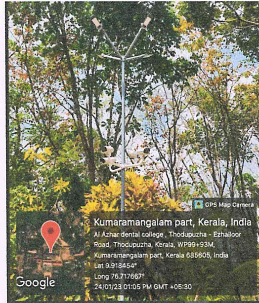
CCTV installed in Dental College
